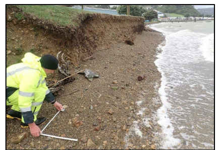
Eroding margin along Titahi Bay Road, western Onepoto
