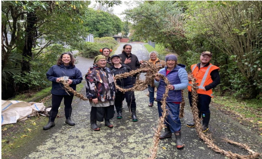
Photo: Te Ātiawa ki Whakarongotai kaimahi with support from Greater Wellington Fish Passage team installing woven natural fibre fish ladders to support fish passage in the Kākāriki stream. Source: Kāpiti Coast District Council
