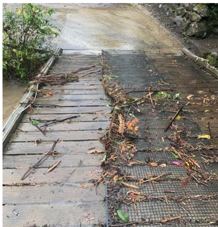
Figure 3 Vehicle bridge along Blue Mountains Road showing debris collected from flood waters overtopping bridge during the storm on 26 August 2024
