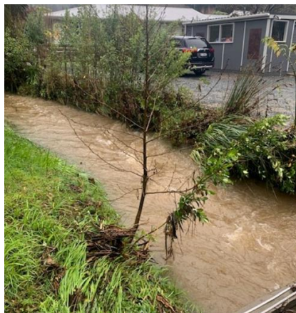
Figure 4 Flood water shown downstream of the Pinehaven culvert just after the peak of the 26 August 2024 storm event
