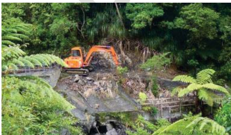
Caption: Orongorongo River track and pipeline repair works 2005. With severe rain events expected to become more frequent, works to strengthen and reinforce assets such as access tracks and water pipelines are required. (Images: GWRC collection)
