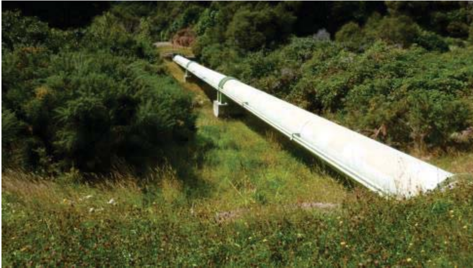
Caption: Raw water supply pipeline upstream of the Wainuiomata Water Treatment Plant
