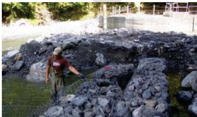
Caption: River bank and asset protection measures such as gabion rock baskets are utilised as flood and erosion stabilisation measures. (Image: GWRC collection)
