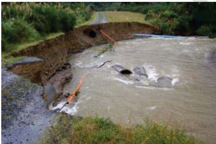
Caption: Heavy erosion of an access road and broken water supply pipe and power cable after a storm in the Wainuiomata catchment downstream of the intake in 2005.
