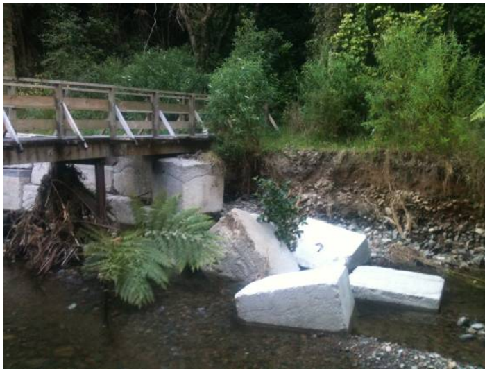
Battle Hill Bridge block damage
