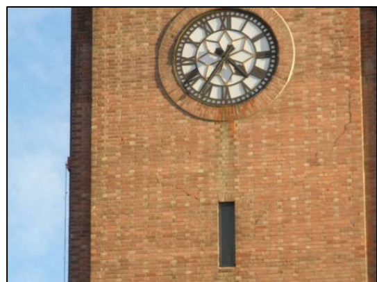
Clock tower of the previous Christchurch Railway Station, note cracking. Photo: M. Kennedy
