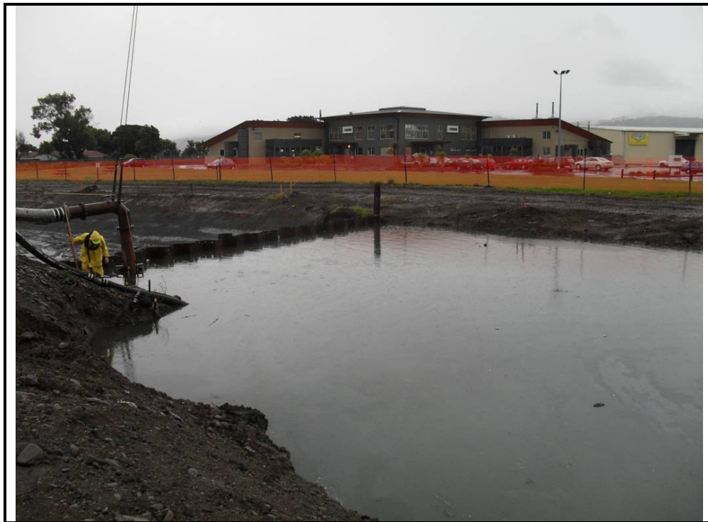
Photograph 2: Cell A during heavy rainfall on 18 November 2009.
