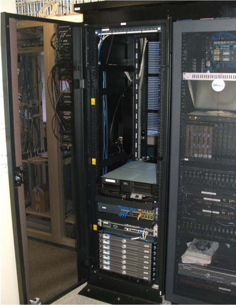
Fig 10.1: The RTPi central control and management system server, recently commissioned and housed in Kordia networks dedicated facility at Avalon
