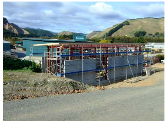
New Substation building in Waikanae
