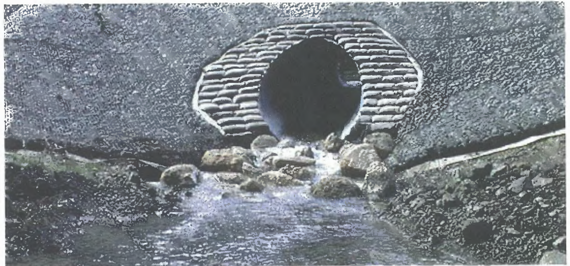
Sandbags and rock placed around the outlet of this culvert help prevent erosion
