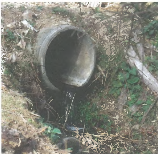
Fish can't migrate up a "perched" culvert
