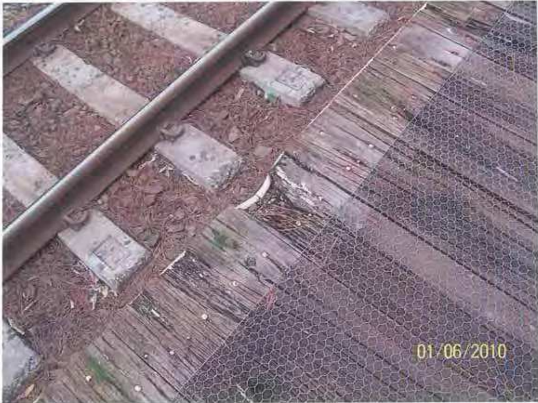
Photo 9 – Up platform timber edge condition
