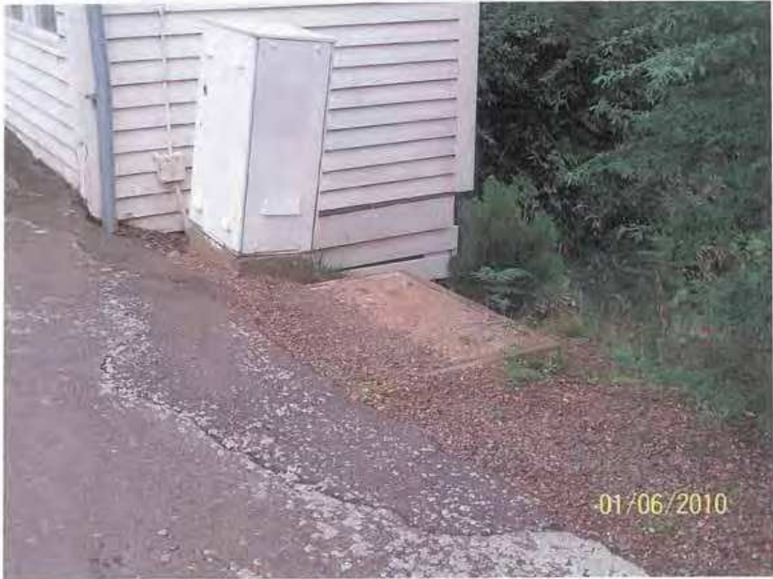
Photo 5 – Up platform surface defect and montrose box
