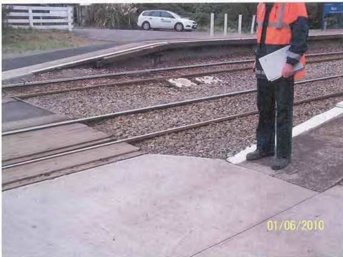
Photo 12– Level crossing devoid of limit lines or TSI's
