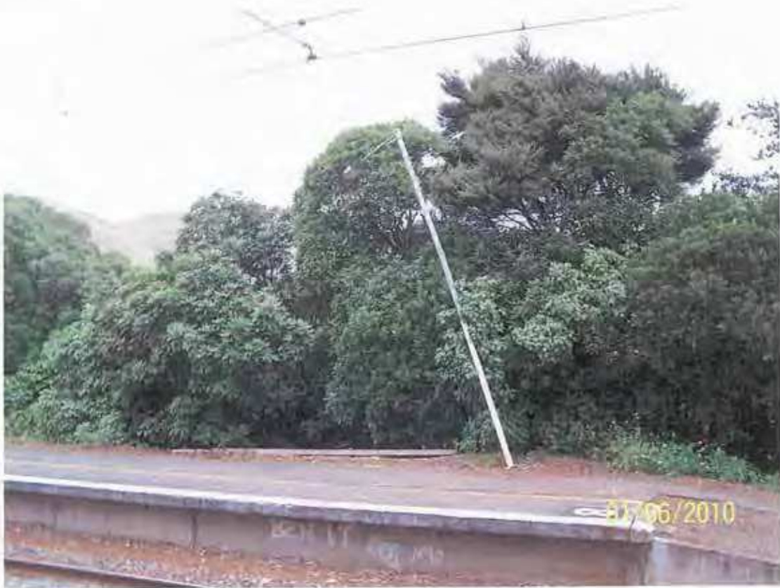
Photo 10 – Down platform lighting mast and damage platform edge
