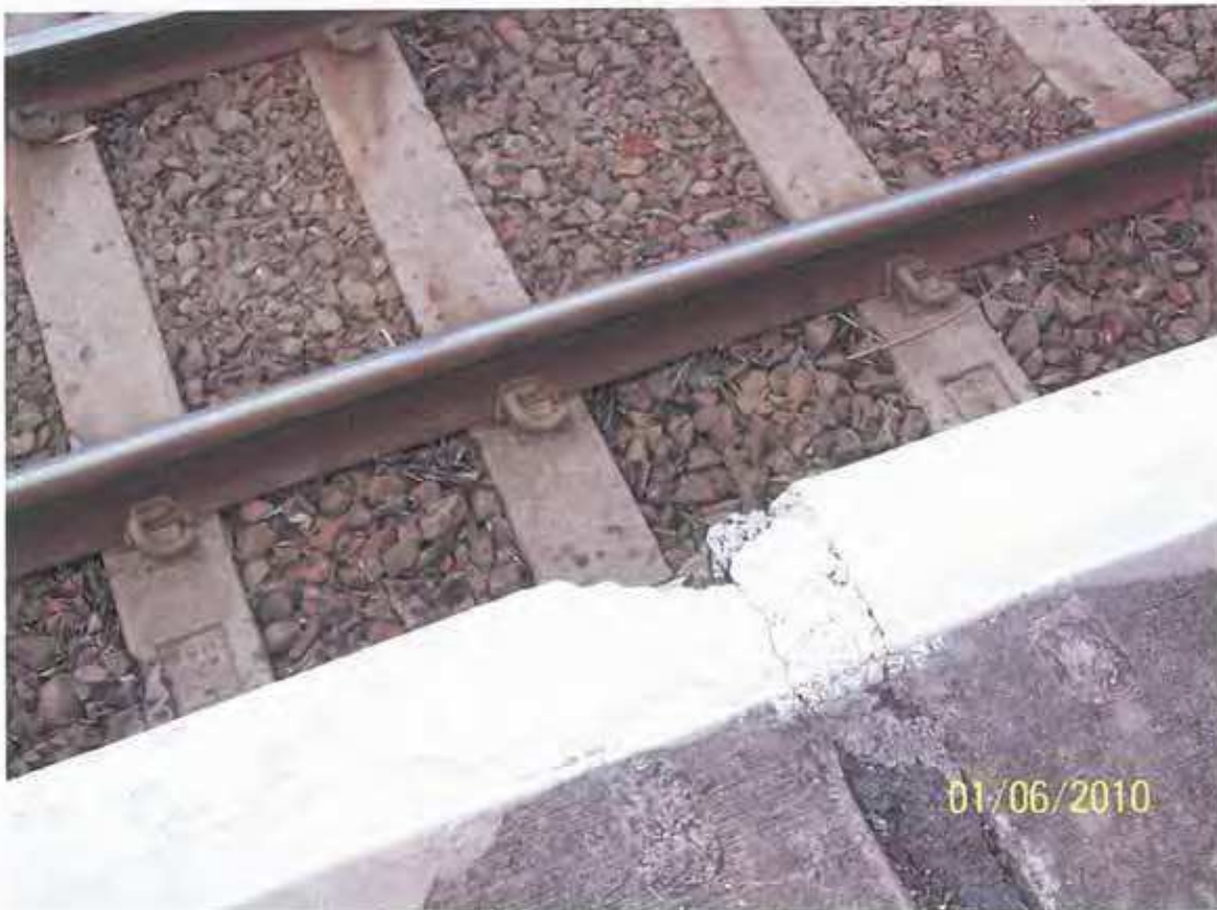
Photo 4 – Up platform edge damage
