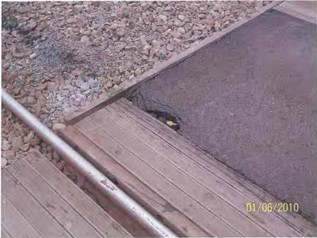
Photo 15 – Level crossing surface defect
