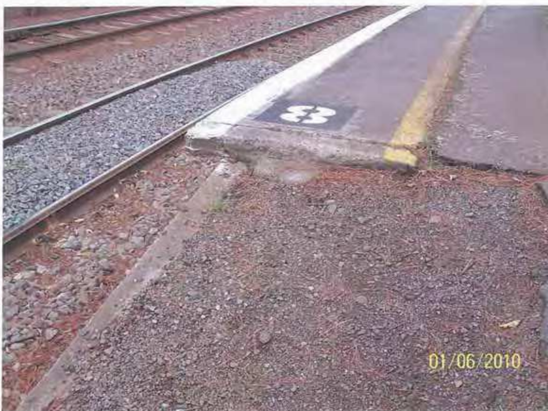
Photo 18 – Down platform southern end – Platform defect
