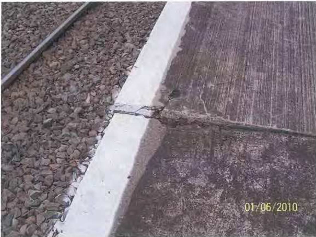
Photo 13 – Up platform northern end – misaligned transition
