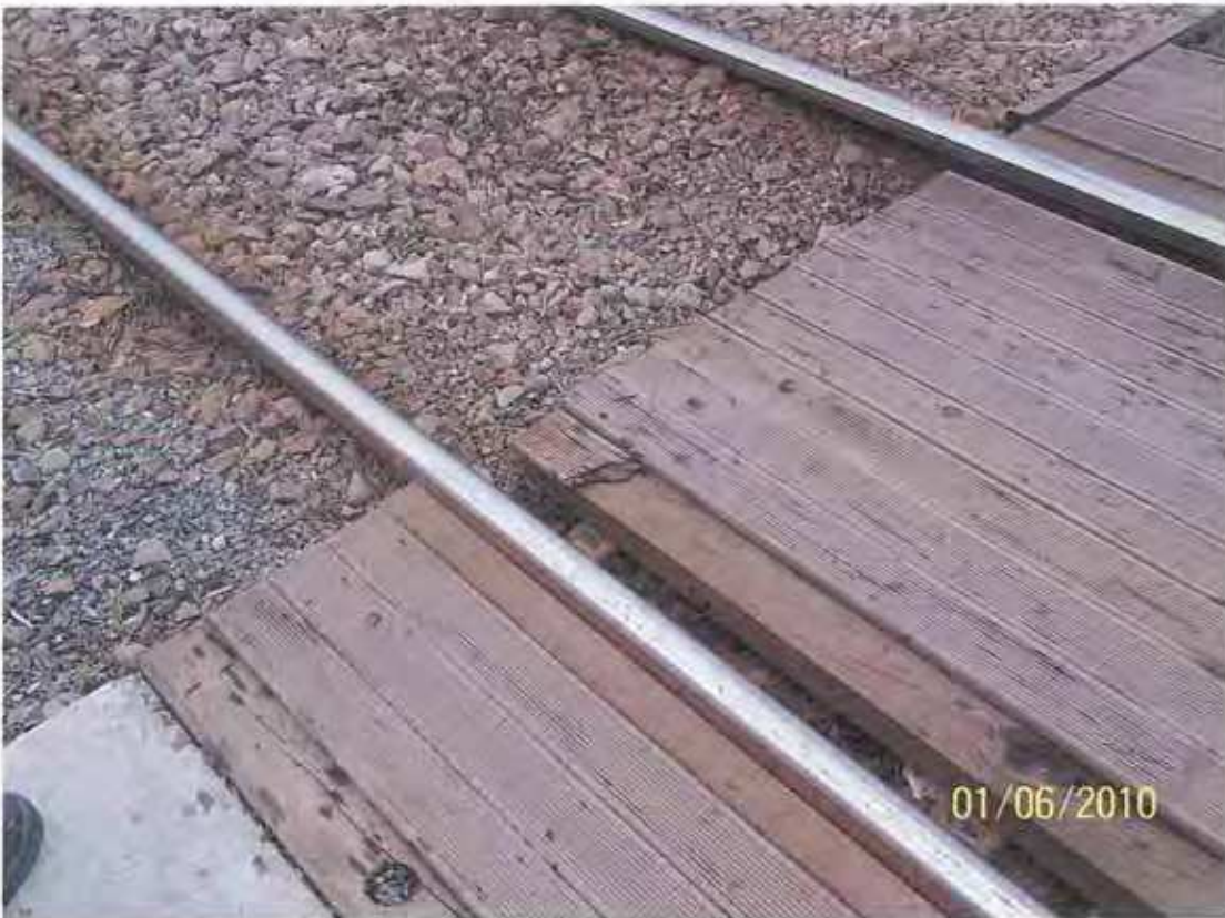
Photo 14 – Level crossing damage and trip hazards
