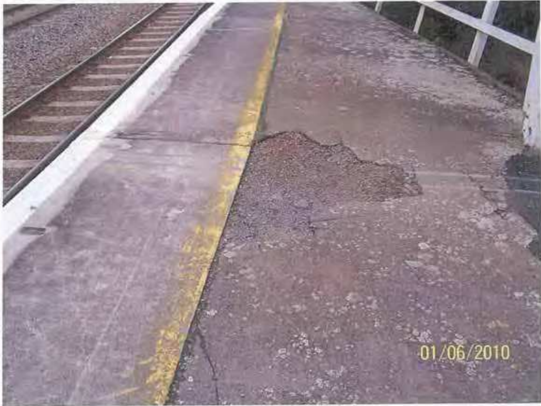
Photo 7 – Up platform surface defect
