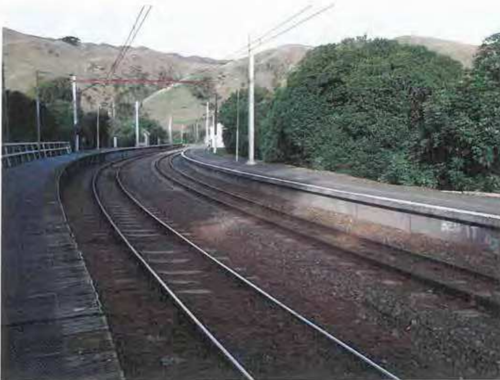
Photo 1: Looking southeast with the Up main on the left with the timber deck section in the foreground
