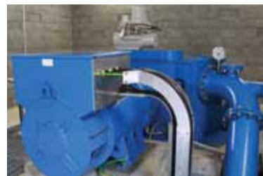
The new hydro-electricity generator
