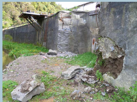
Damaged lower dam
